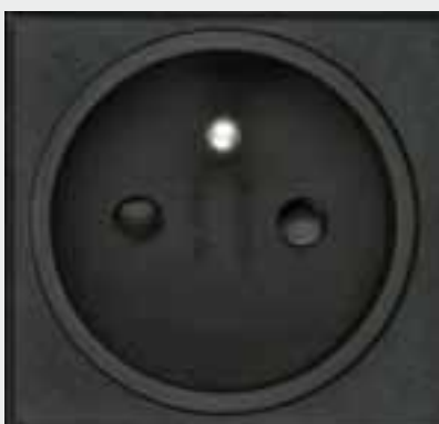
With central earth pole
